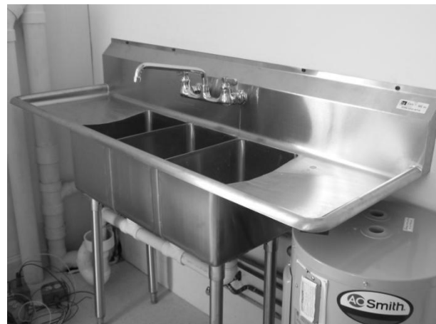
Catering sink and water heater
