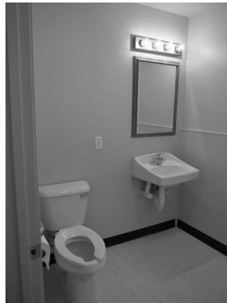
Additional ADA-compliant restroom
