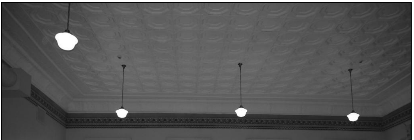
Newly restored metal tile ceiling, school house lights and period-correct wallpaper frieze
